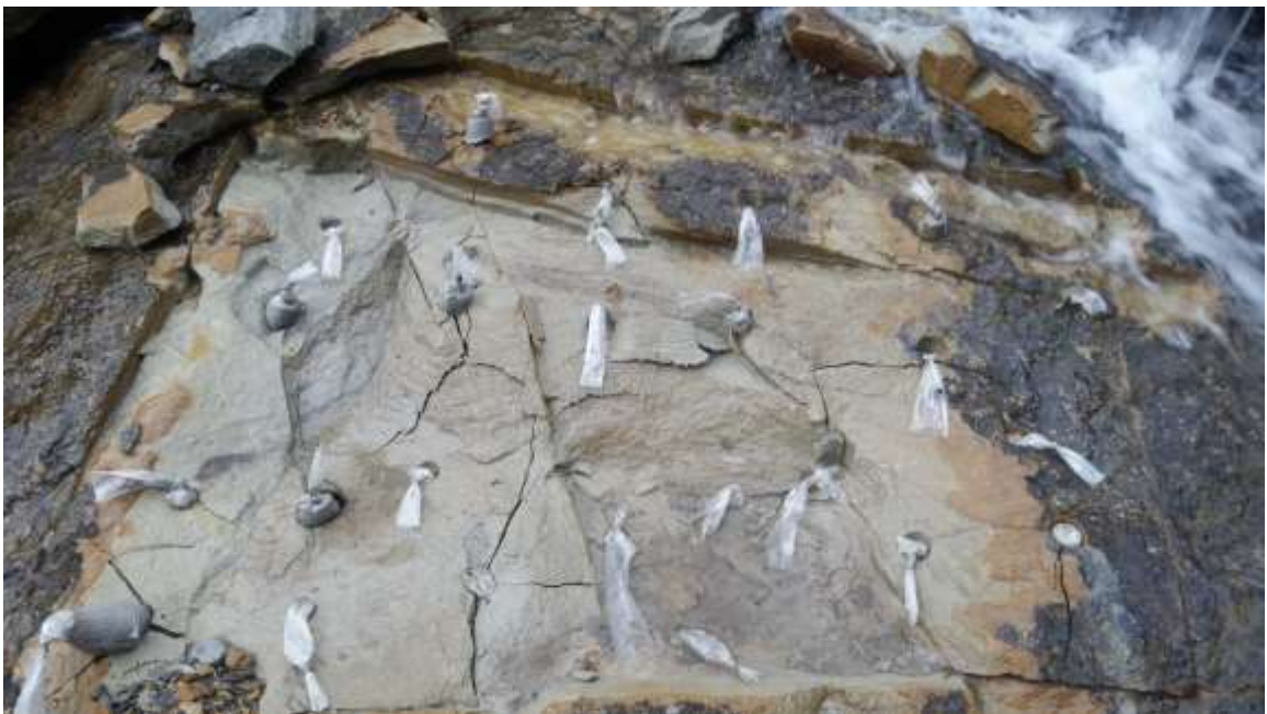
Photo 14. After successful pressure fracturing of the bedrock debris could be removed using a demolition hammer, pry bars, or by hand.
