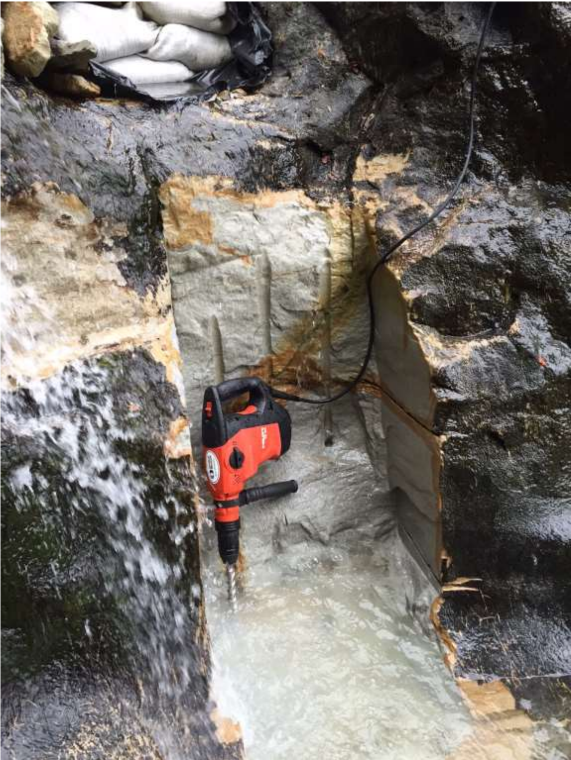
Photo 11. Drilling holes for more pressure fracturing beneath an area that was previously successfully fractured by Dexpan. Relief cuts on either side of the excavation were made with a rock chain saw which proved very effective.
