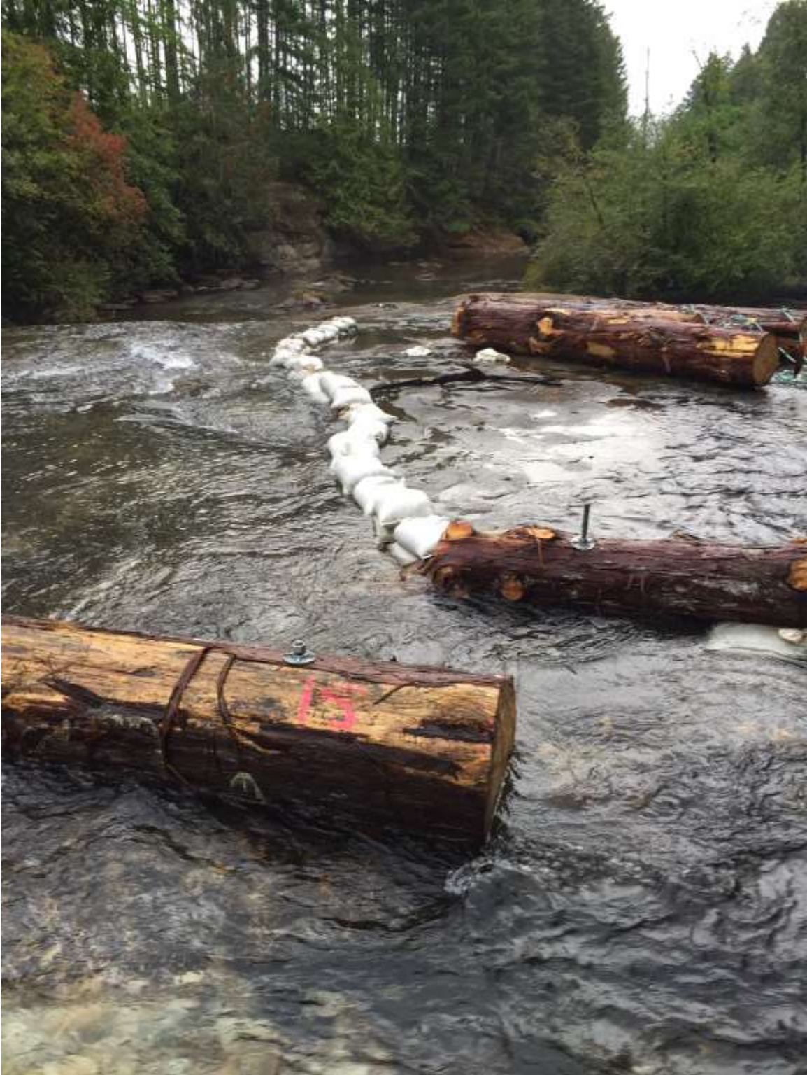
Photo 3. Sand bags placed at a 45° to the direction of flow effectively redirecting the flow of the Quinsam River.
