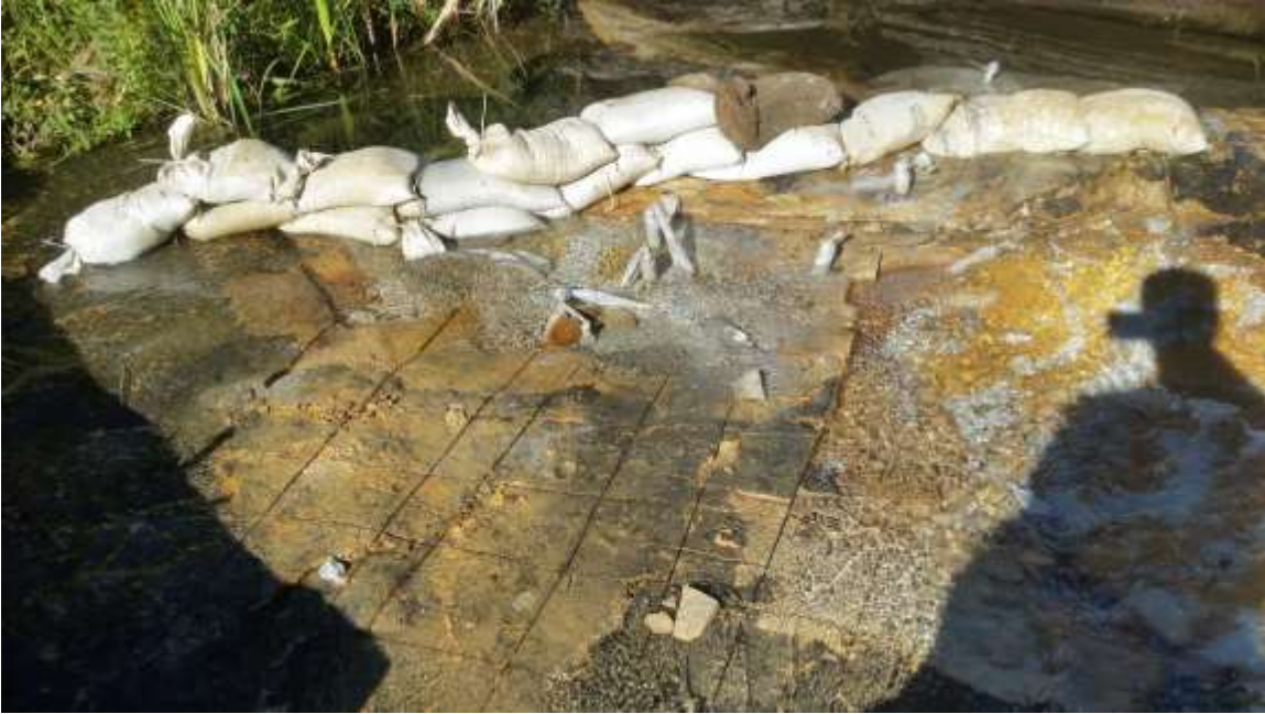
Photo 10. Relief cuts in the bedrock improved the effectiveness of the Dexpan. Note the plastic sleeves with the dexpan agent being utilized in standing water. This particular fracture was very successful.
