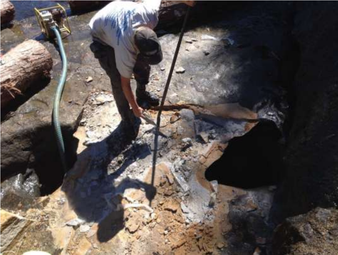
Photo 5. Dewatering pump being used effectively to draw down the water level at a localized work area.
