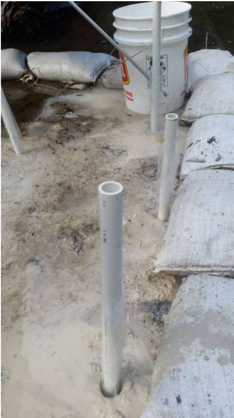
Photo 12. Holes drilled and prepared for the pouring of Dexpan. PVC tubing allowed for efficient pouring of Dexpan slurry into the plastic hole liners.
