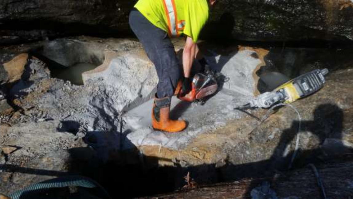
Photo 15. Relief cuts made with a line saw improved the efficiency of the demolition hammer.
