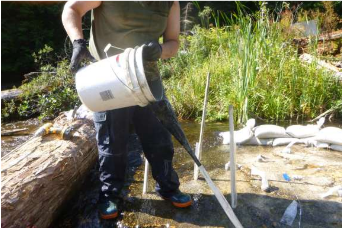
Photo 13. Dexpan was mixed in a 5 gallon bucket and poured into the PVC tubing with a funnel.
