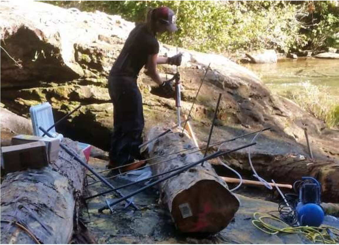
Photo 8. Epoxy being applied through flexible plastic tubing to an anchor hole in the bedrock beneath a log.
