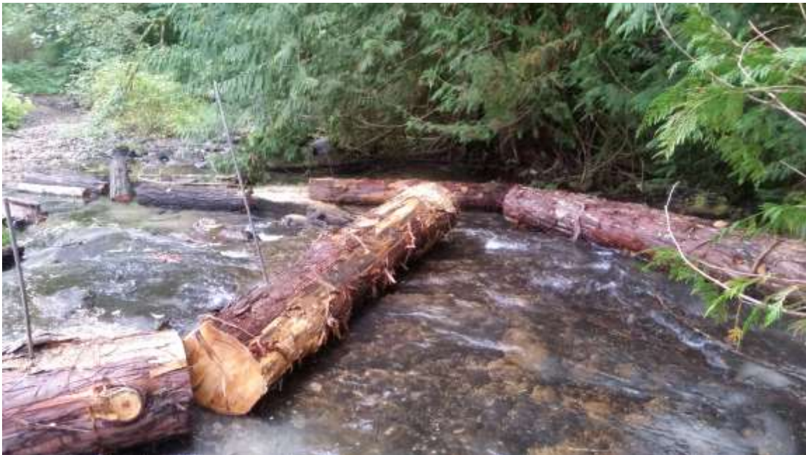
Photo 7. Logs being held in position with rebar while they are prepared for anchoring.
