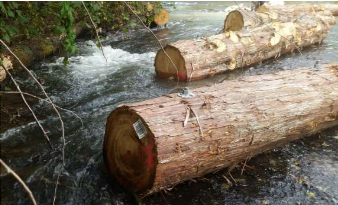
Photo 9. Fully anchored log with epoxied galvanized threaded rod, washer and nut attached.
