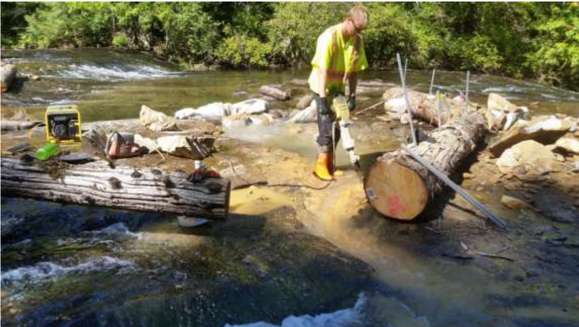
Photo 16. Mechanical fracturing of rock was possible with some water flow through the site.
